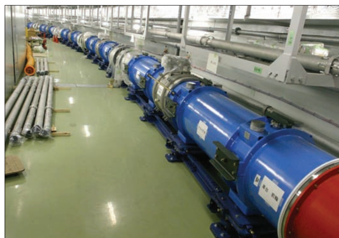
Superconducting combined function magnets in the arc of the primary beam line for the T2K facility. (All photos courtesy KEK.)
