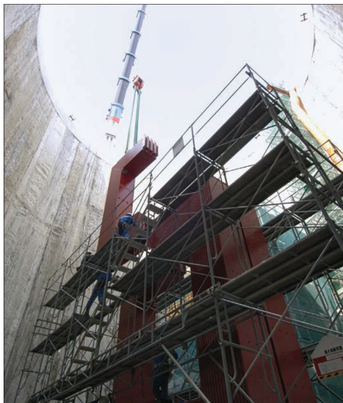
Installation of the sections of the magnet yoke familiar from UA1 and NOMAD gets under way in the neutrino monitor pit.
